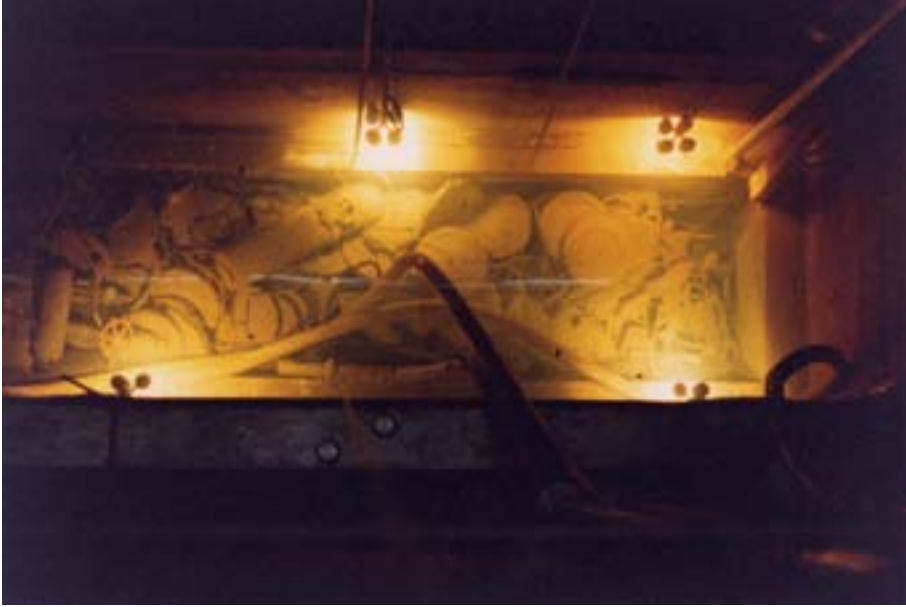
FIG. 24. Wastes piled up in the high activity pit at the Garigliano nuclear power plant, Italy.
