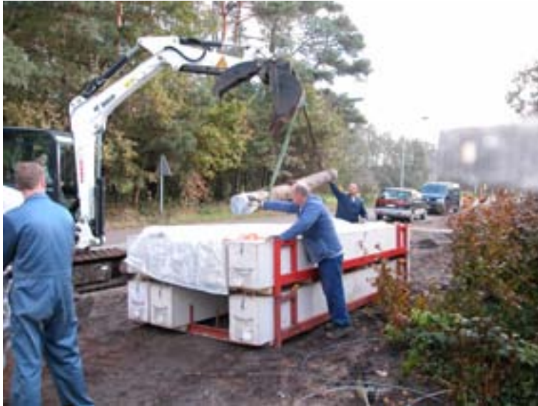
FIG. I-6. Underground pipeline decommissioning in Belgium: sealing of the pipe ducts. Courtesy: Belgoprocess.
