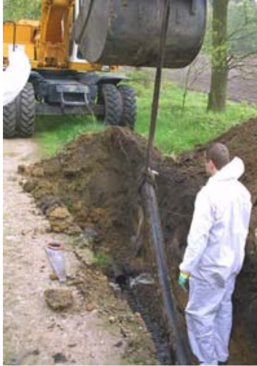
FIG. X-1. Excavation of a pipe in connection with Molse Nete discharge line decommissioning, Belgium.
