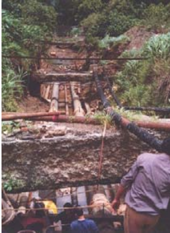
FIG. VIII-3. View of the underground pipes near completion of work at the Cirus reactor, India.
