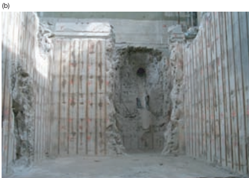
FIG. III-2. An embedded pipe at Vandellós 1 nuclear power plant before (a) and after (b) removal.
