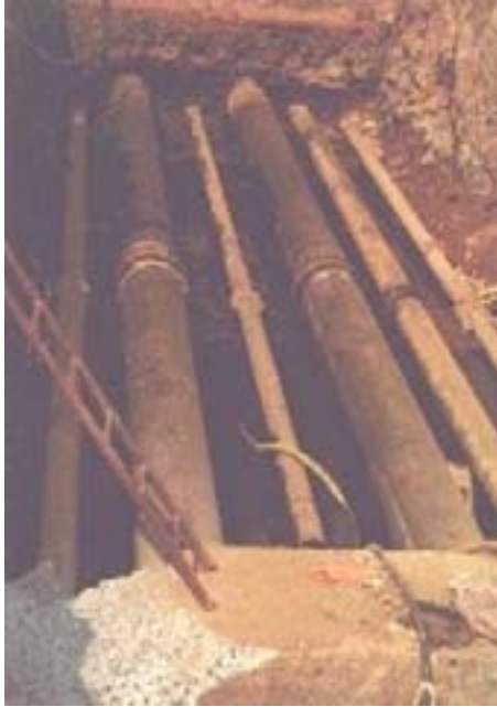
FIG. VIII-1. View of underground pipes at the Cirus reactor, India.
