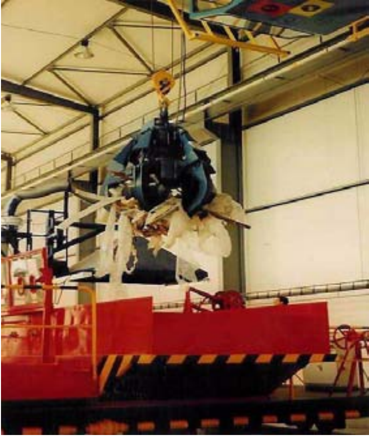
FIG. VII-12. Retrieval of solid wastes from the SRWSF tanks at the A-1 nuclear power plant at Jaslovské Bohunice.
