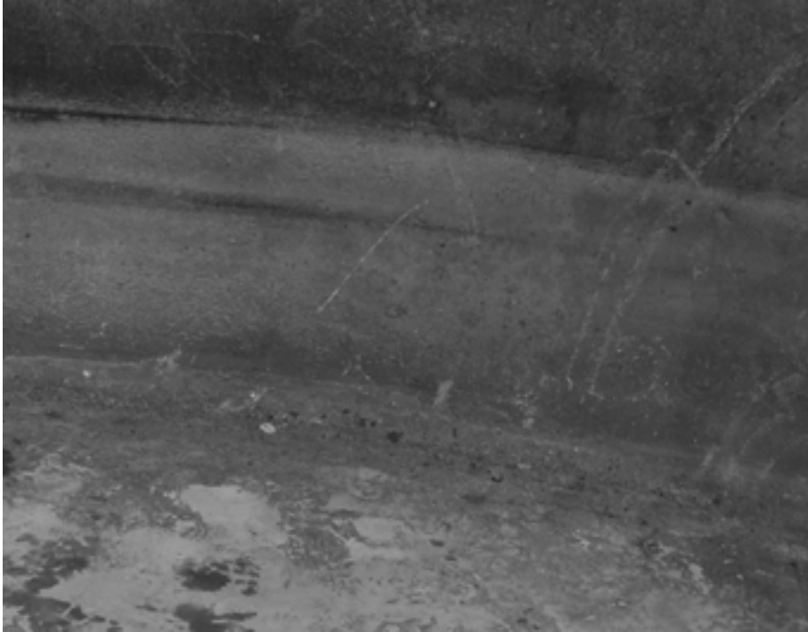
FIG. VII-7. Example of the state after decontamination of the surface of an underground tank at the A-1 nuclear power plant at Jaslovské Bohunice.
