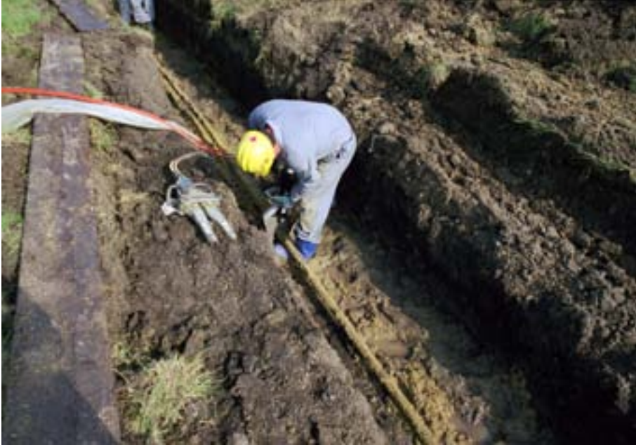
FIG. 12. Dismantling of a buried pipe using hydraulic cutters at the ANL pneumatic transfer tube project, Argonne, Illinois, USA. Courtesy: Argonne National Laboratory, managed and operated by the University of Chicago for the USDOE under Contract No. W-31-109-ENG-38.
