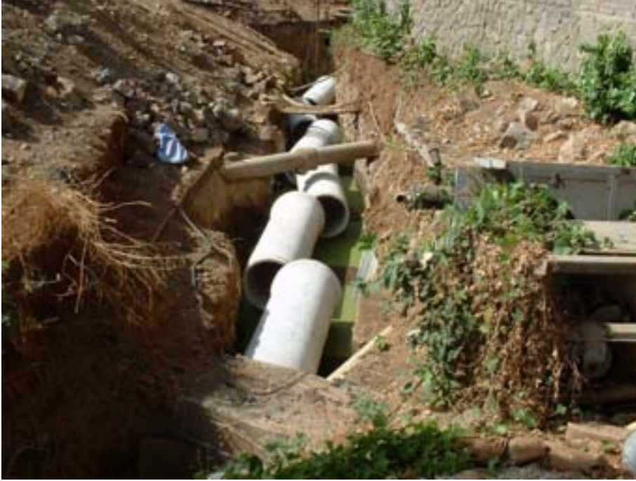
FIG. VIII-4. New underground ventilation concrete pipes being laid after removal of the old pipes at the Cirus reactor, India.
