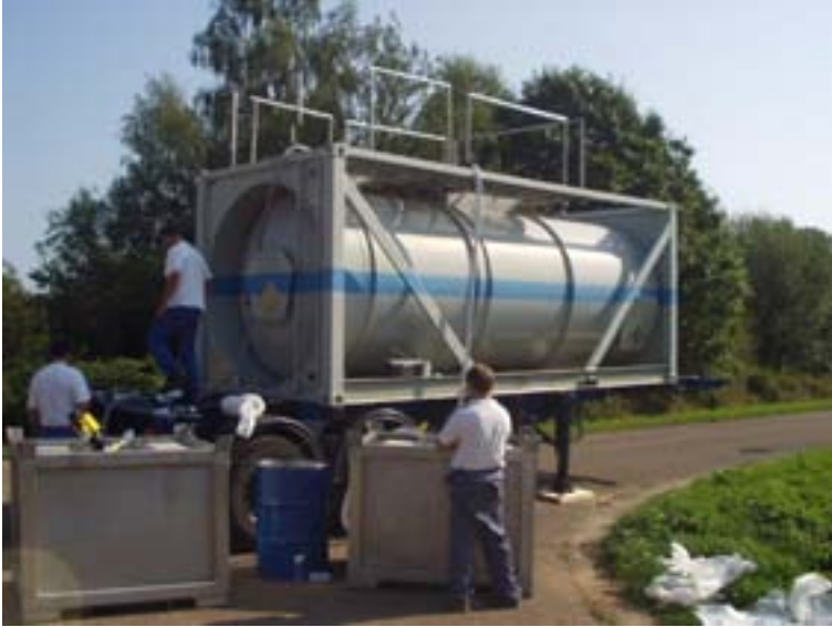
FIG. I-2. Underground pipeline decommissioning in Belgium: dewatering of the discharge line. Courtesy: Belgoprocess.
