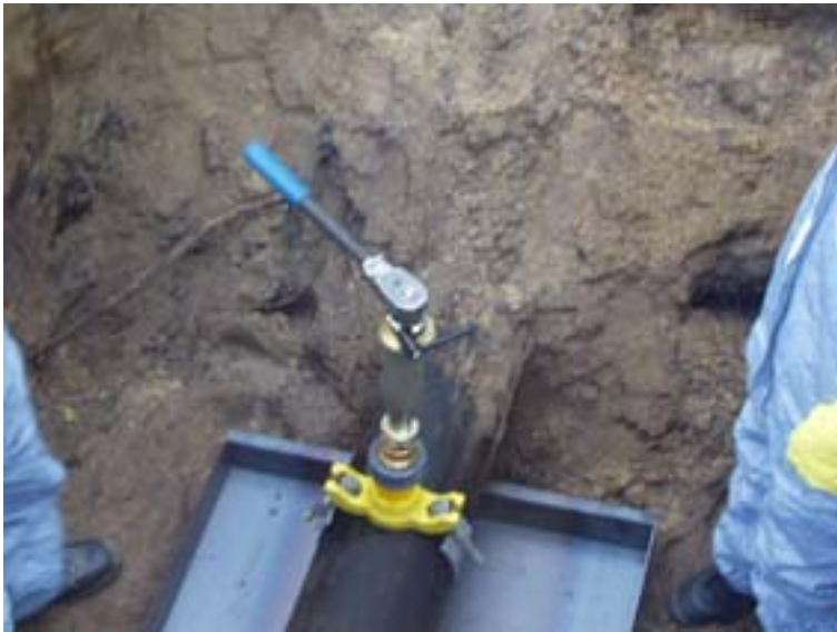
FIG. I-4. Underground pipeline decommissioning in Belgium: boring holes in the discharge line. Courtesy: Belgoprocess.
