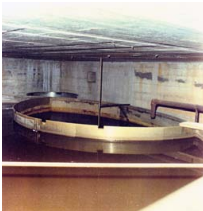
FIG. 22. An underground tank for storing resins at the Garigliano nuclear power plant, Italy. Courtesy: AnsaldoEnergia.
