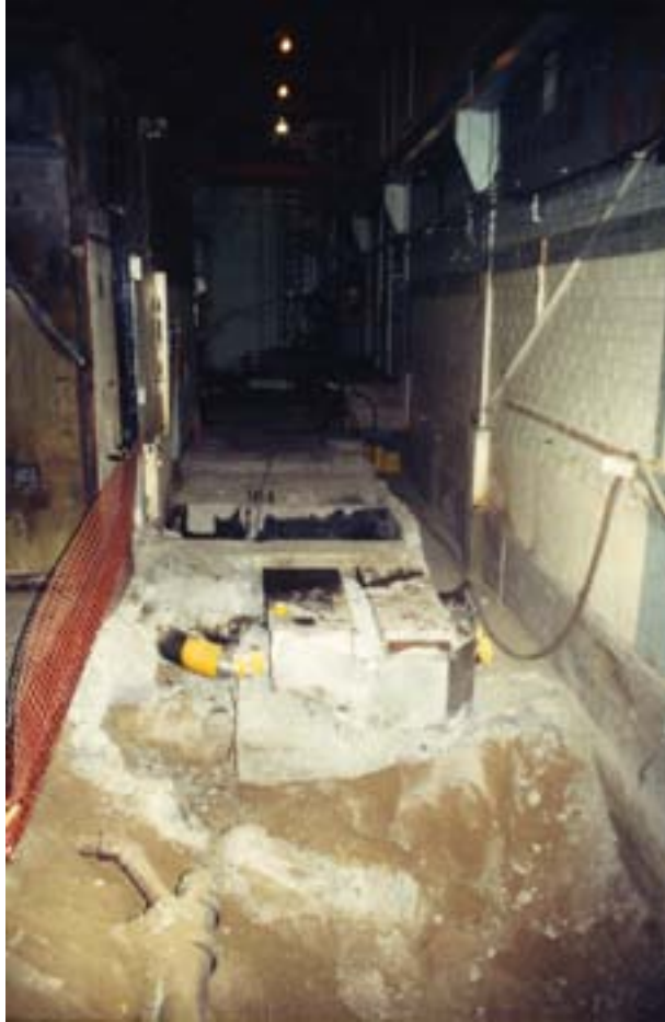
FIG. 4. Hot cell dismantling: removal of various embedded process systems for servicing the cell at the radioisotope production facility at Tunney's Pasture, Ottawa, Canada. Courtesy: Atomic Energy of Canada Limited.
