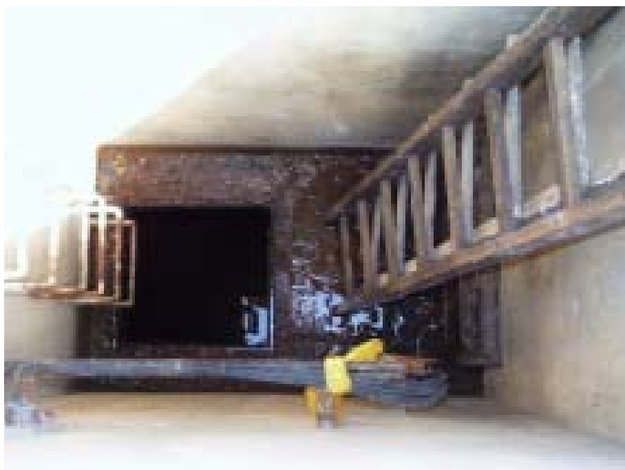
FIG. VII-3. Example of the situation in an inspection shaft at the A-1 nuclear power plant at Jaslovské Bohunice.
