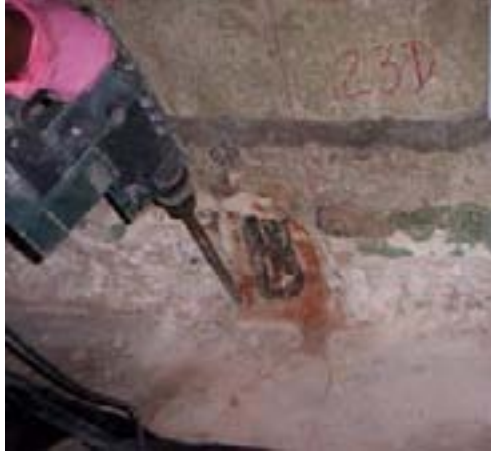
FIG. IX-9. Pipe embedded in a wall at INOR, Havana.
