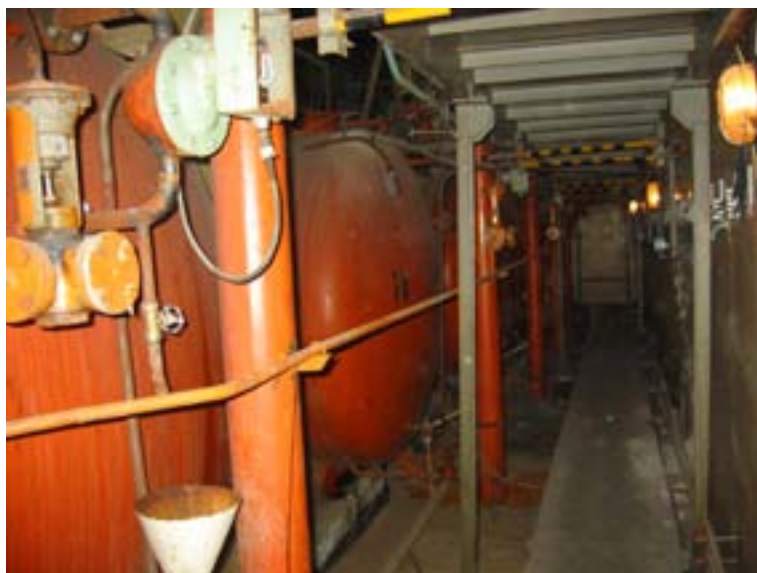
FIG. II-5. The underground bunker with a storage tank in building 241 at NRI in the Czech Republic.
