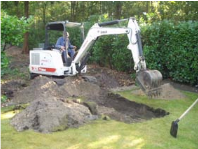
FIG. I-3. Underground pipeline decommissioning in Belgium: removal of soil above the discharge line. Courtesy: Belgoprocess.
