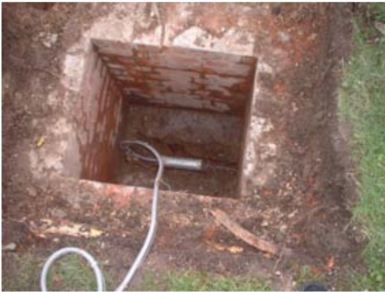
FIG. V-2. The pipe survey equipment in use at Harwell, UK.
