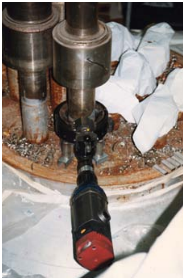
FIG. 10. Cutting reactor head standpipes using an orbital cutter with a lathe at the BR-3 Mol decommissioning project, Belgium. Courtesy: Studiecentrum voor Kernenergie – Centre d'Étude de l'Énergie Nucléaire (SCK·CEN).
