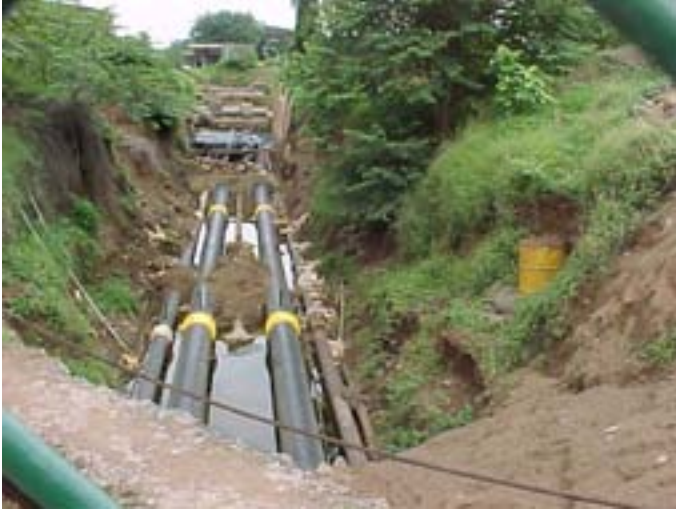
FIG. 15. View of subsoil primary coolant pipes with cold self-adhesive bituminous tapes newly applied before backfilling at the Cirus reactor, India.
