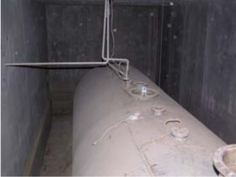
FIG. II-6. Storage tanks in building 241 at NRI in the Czech Republic.
