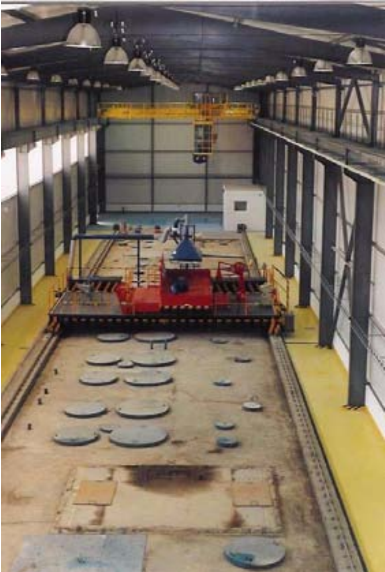
FIG. VII-10. The solid radioactive waste storage facility at the A-1 nuclear power plant at Jaslovské Bohunice.
