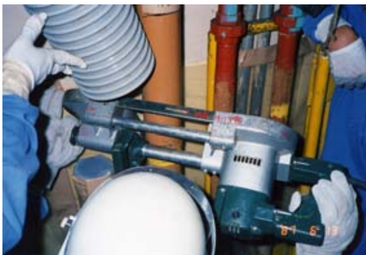
FIG. 9. Cutting of pipes using a bandsaw at the JPDR (Japan Power Demonstration Reactor) commissioning project, Japan. Courtesy: Japan Atomic Energy Research Institute.
