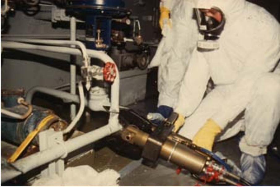
FIG. 11. Cutting pipes with diameters of up to 2 in (5 cm) using hydraulic shears at the Mol decommissioning project, Belgium. Courtesy: SCK·CEN.
