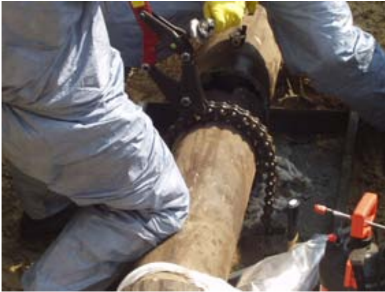
FIG. I-5. Underground pipeline decommissioning in Belgium: the pipe cutter used for cutting asbestos cement pipelines. Courtesy: Belgoprocess.
