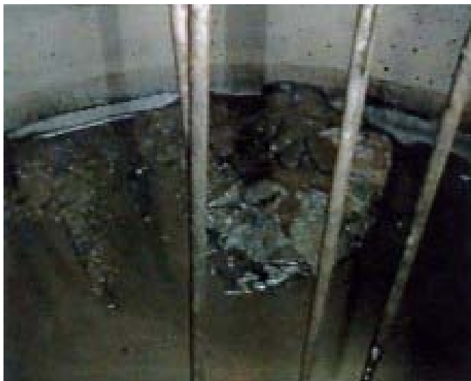
FIG. VII-2. Example of the situation at the bottom of tanks at the A-1 nuclear power plant at Jaslovské Bohunice.
