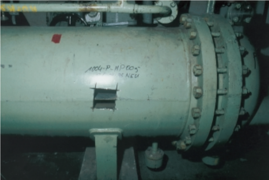
FIG. 10. Heissdampfreaktor (HDR) decommissioning project: a component where a sample was cut from the shell for characterization purposes.
