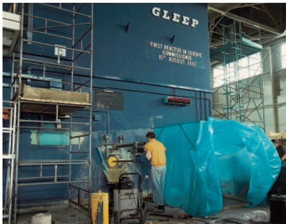
FIG. 9. GLEEP reactor, UK (graphite reactor): taking concrete samples from the biological shield and preparing access arrangements for the defuelling machine.
