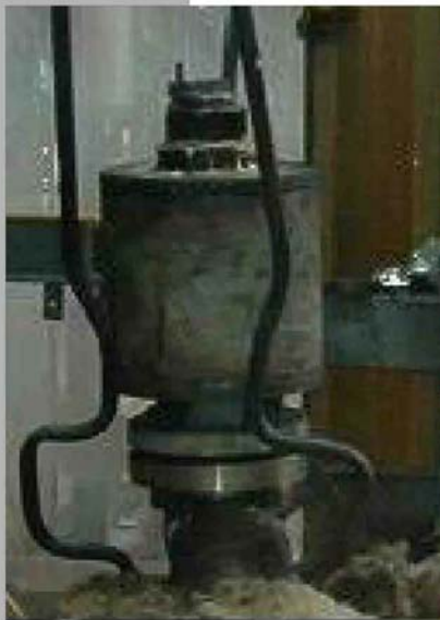
SERB-HP-100 Damper for Hydraulic shocks isolated on pump outlet pipe PL1056
